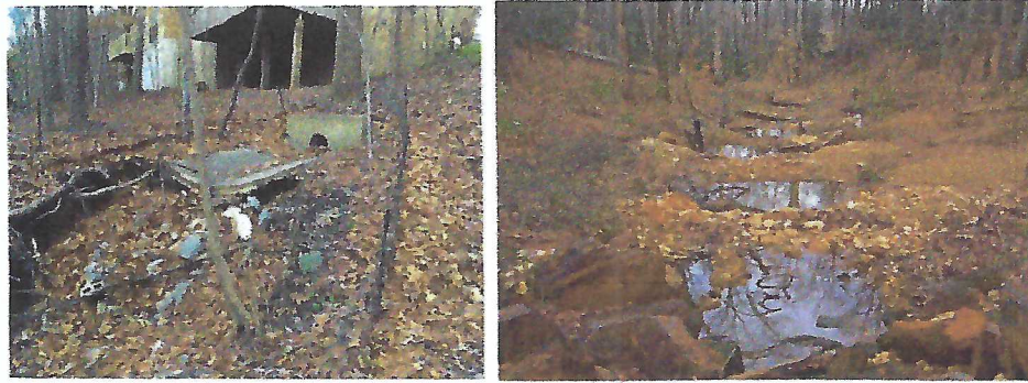
Figure 11. (a) Existing outfall in need of stabilization, and (b) Example step pool stormwater conveyance system.
