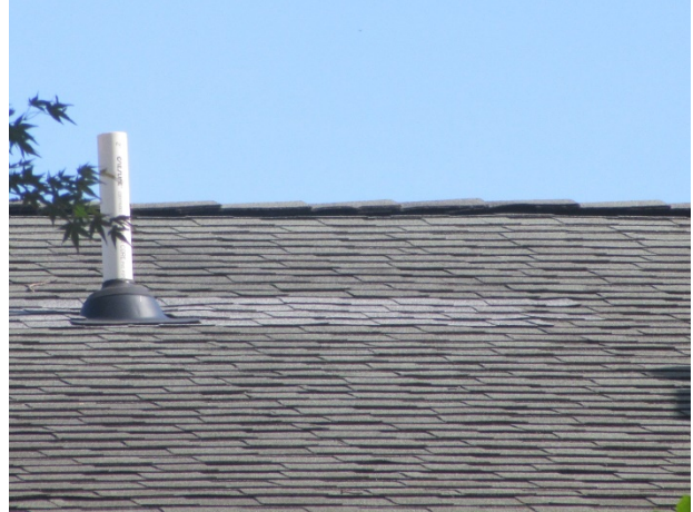
Asphalt shingle roof previous repairs
