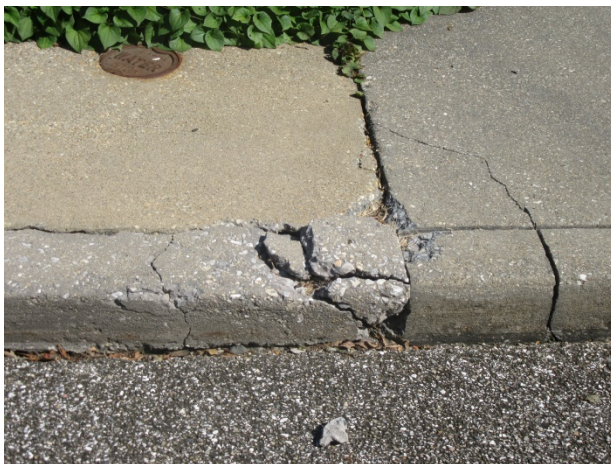
Concrete curb deterioration
