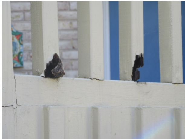
Wood fence deterioration at unit 54
