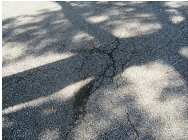
Asphalt pavement cracks and minor deterioration
