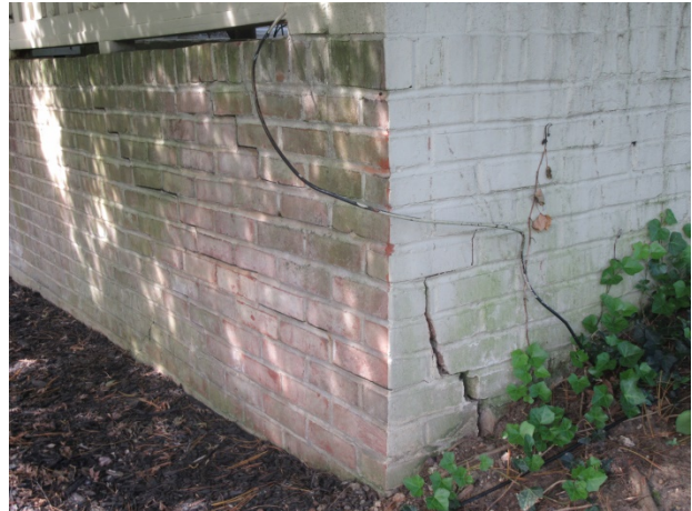
Retaining wall masonry crack
