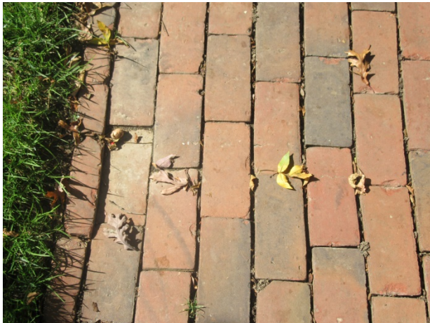
Pavers displacement and vegetation growth
