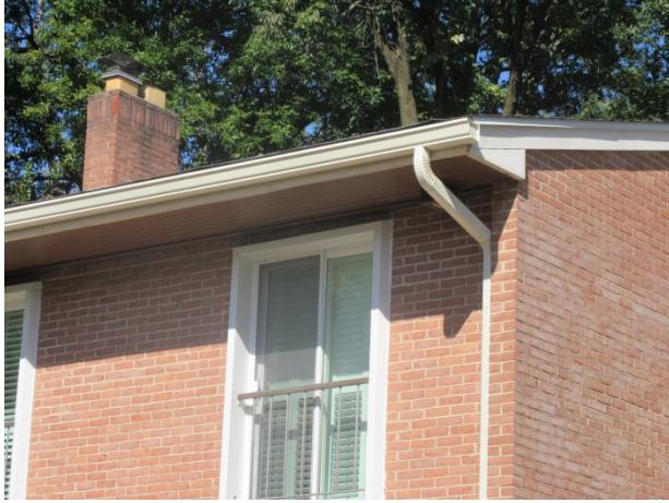
Gutter and downspout assembly
