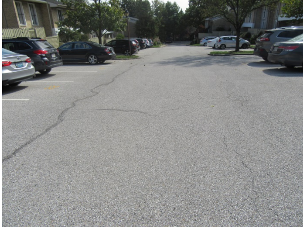
Asphalt pavement; we note minor cracks and previous repairs
