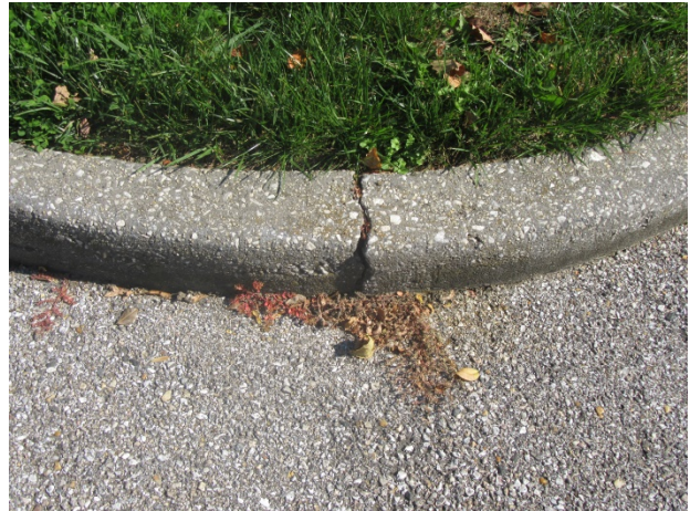
Concrete curb crack
