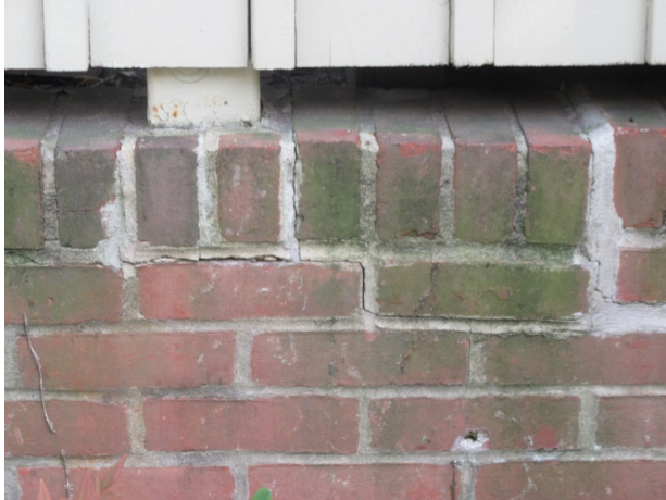
Retaining wall mortar crack
