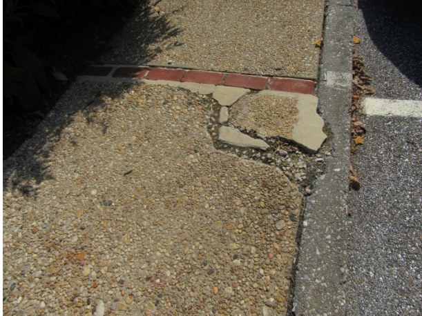
Concrete sidewalk deterioration
