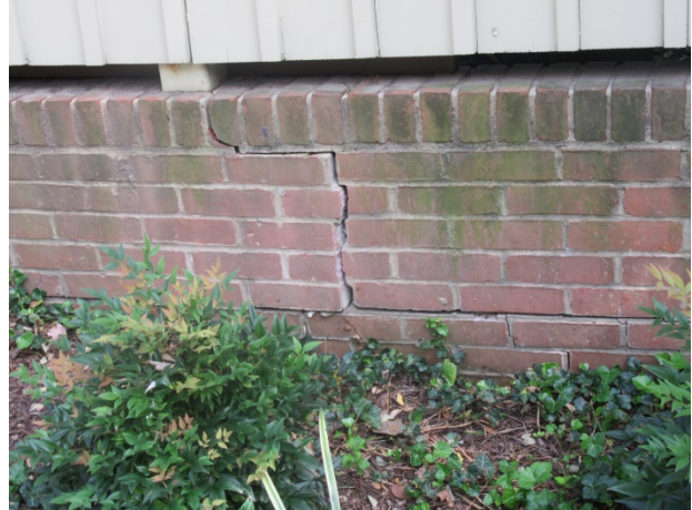
Retaining wall masonry and mortar cracks
