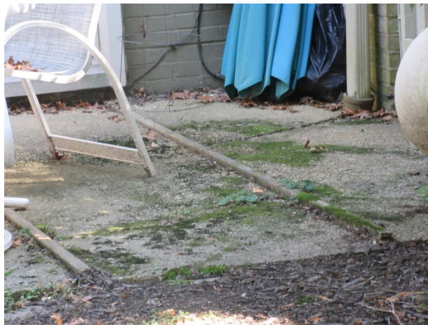
Concrete patio; we note organic growth and deterioration
