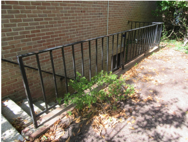
Metal railings; we note rust and finish deterioration
