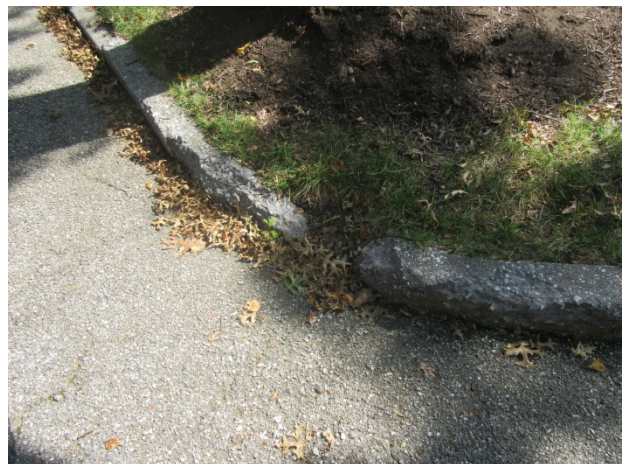
Concrete curb deterioration
