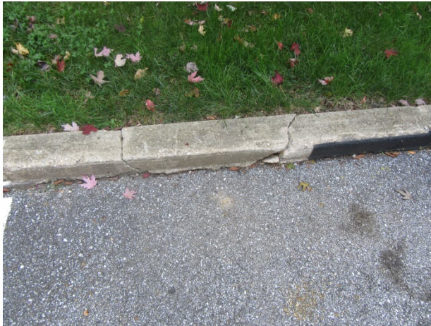
Concrete curb cracks and deterioration
