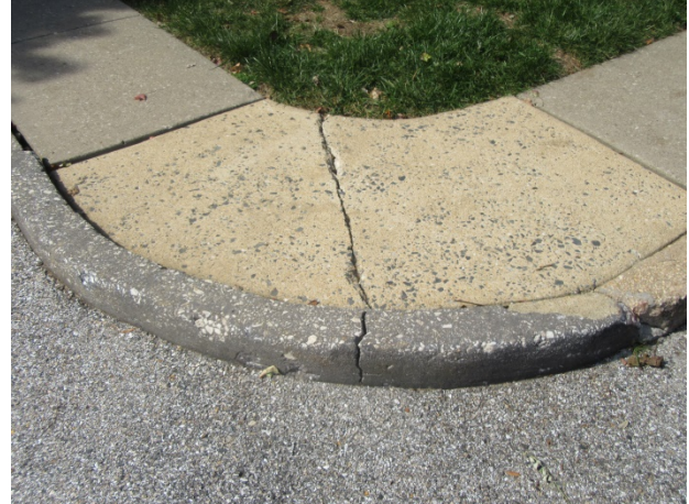
Concrete sidewalk crack and spall
