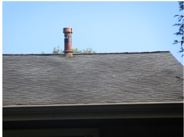
Asphalt shingle roof stains
