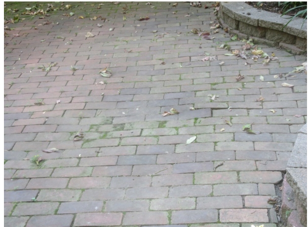
Pavers displacement and organic growth
