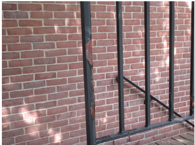
Metal railings rust and finish deterioration
