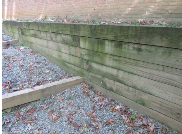
Timber retaining wall organic growth
