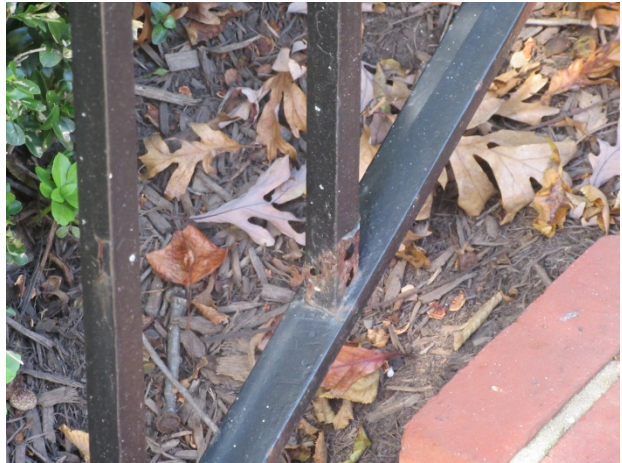
Metal railings rust and deterioration
