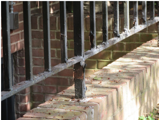
Metal railings rust and finish deterioration
