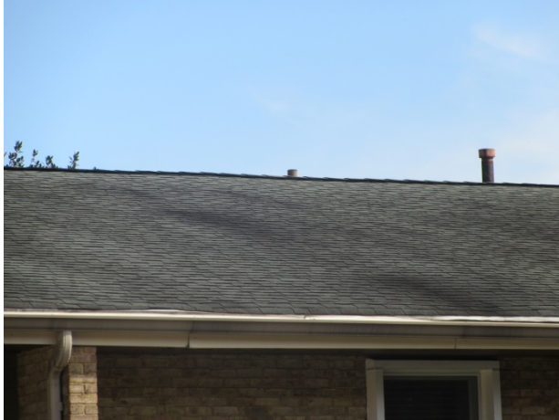
Asphalt shingle roofs stains
