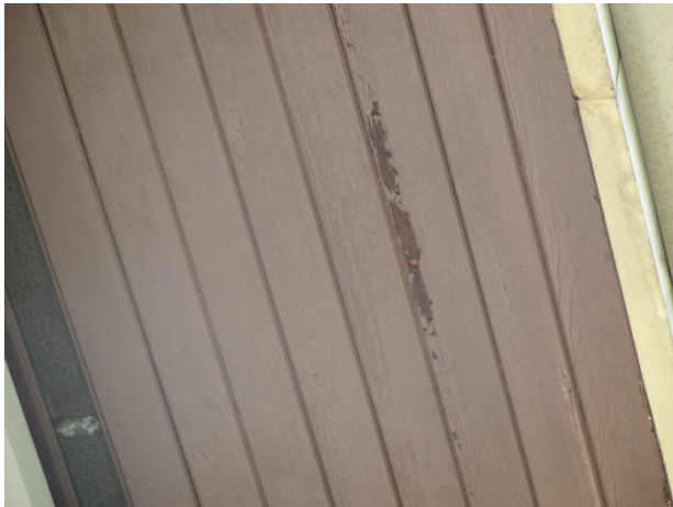
Soffit minor deterioration
