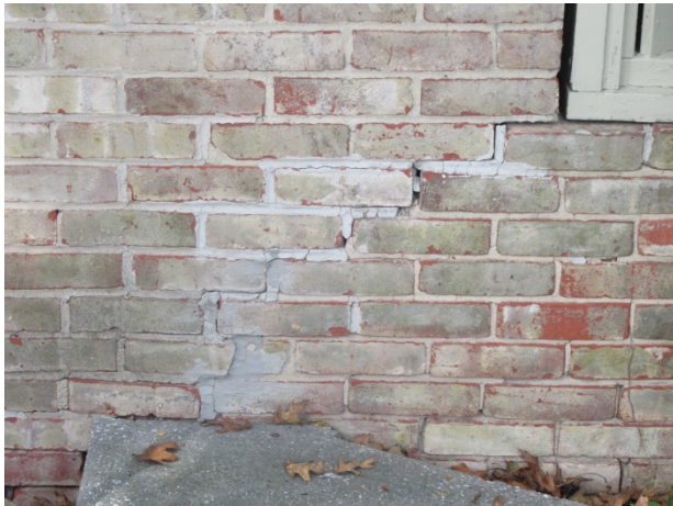
Previous repairs and mortar deterioration
