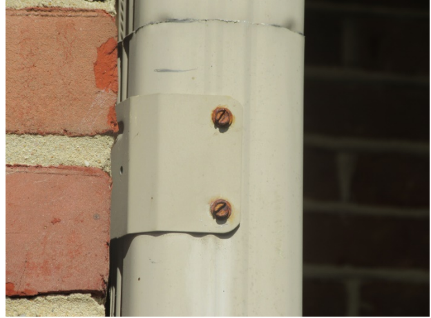
Downspout fastener rust
