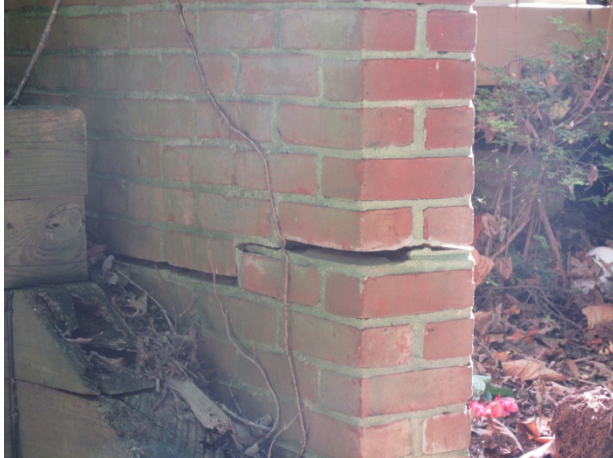
Mortar cracks and deterioration
