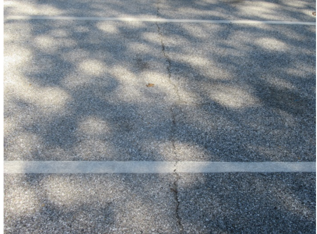
Asphalt pavement cracks
