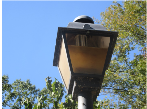
Damaged light fixture at Bouton Court. We assume the Association will replace this light fixture in the near term and fund this activity through the operating budget
