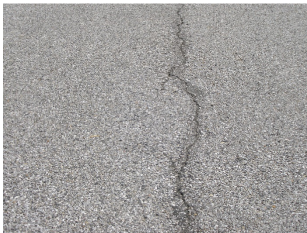
Asphalt pavement crack
