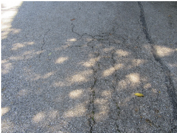
Asphalt pavement cracks, previous repairs, and minor deterioration
