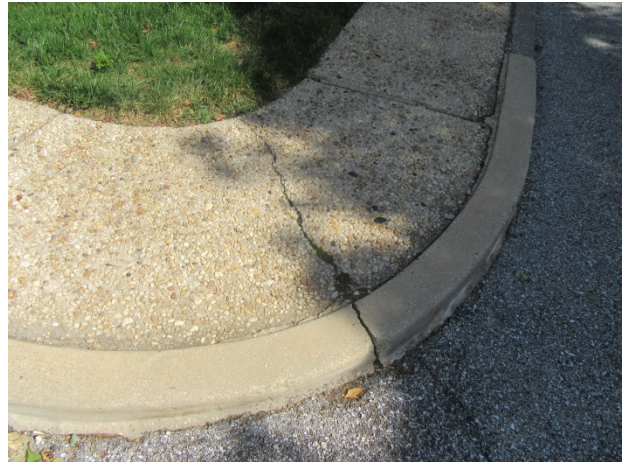
Concrete sidewalk crack
